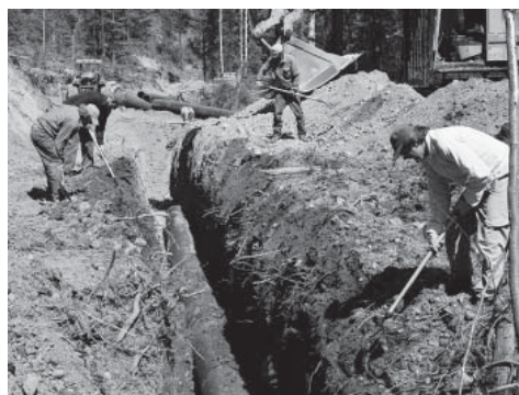
Digging the trench for a new pipeline that will improve the irrigation system at Talking Mtn Ranch and also for our neighbours. Photos by David Pettigrew
